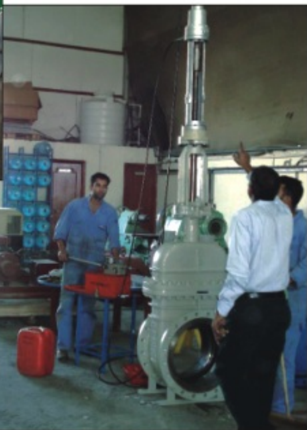
Gate valve stroke checking with hydraulic actuator
